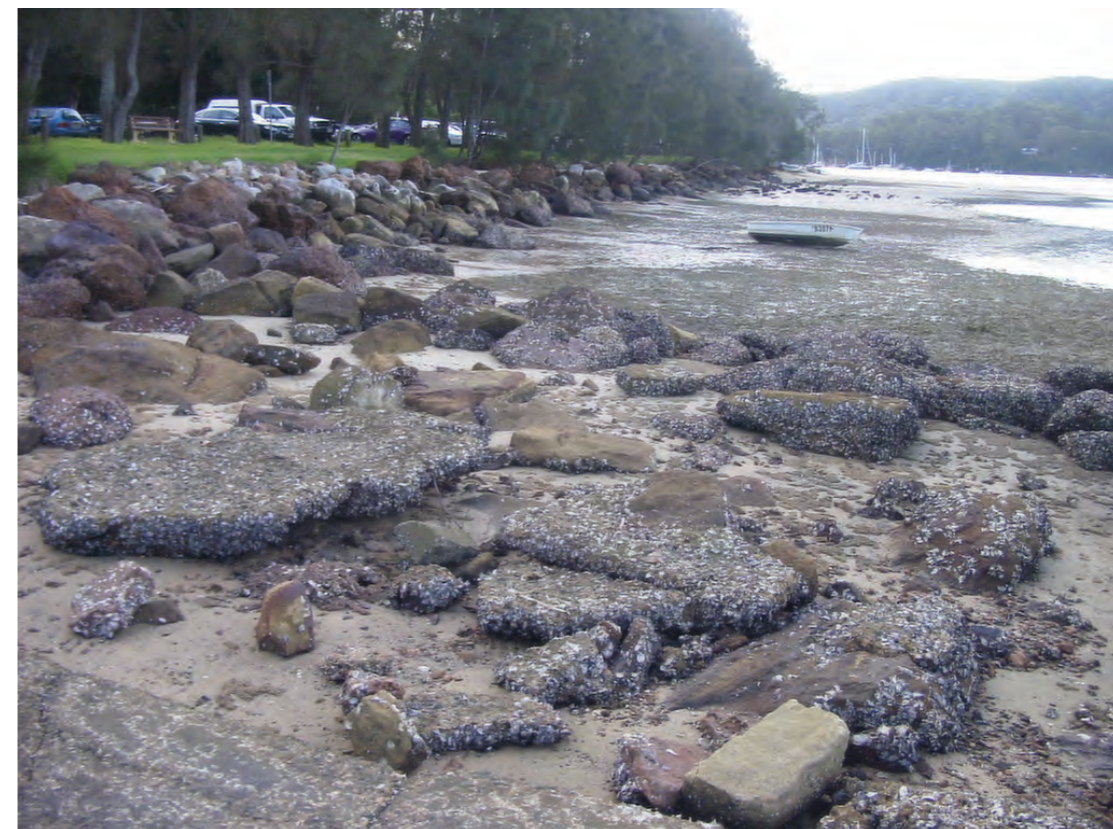
Fig 6 North-eastern face of car park showing loose rubble revetment and loose rock alongside concrete boat ramp (in foreground) plus intertidal sand and mud flat off-shore.
