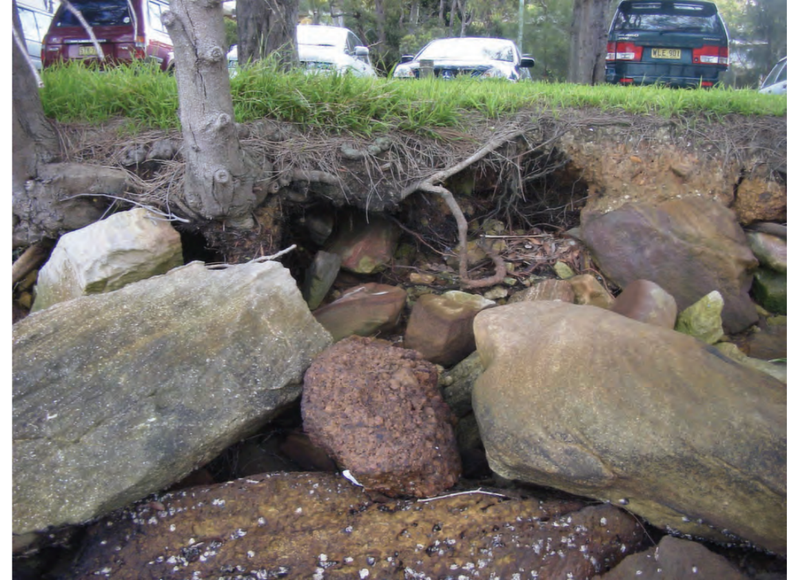
Fig 12 Bank erosion of car park fill, exposing She-oak roots
