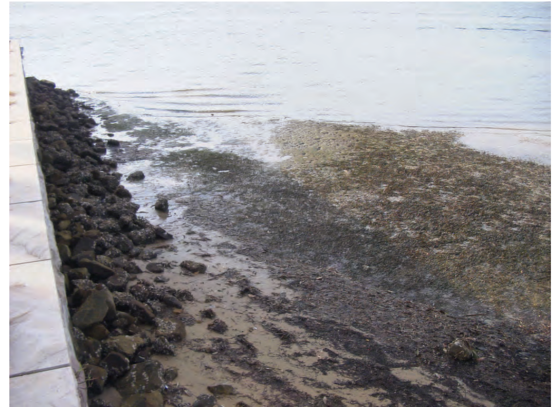
Fig 24 Placement of rock rubble at toe of Seawall (Precinct 2) to provide shallow sub-tidal habitat and shelter.
