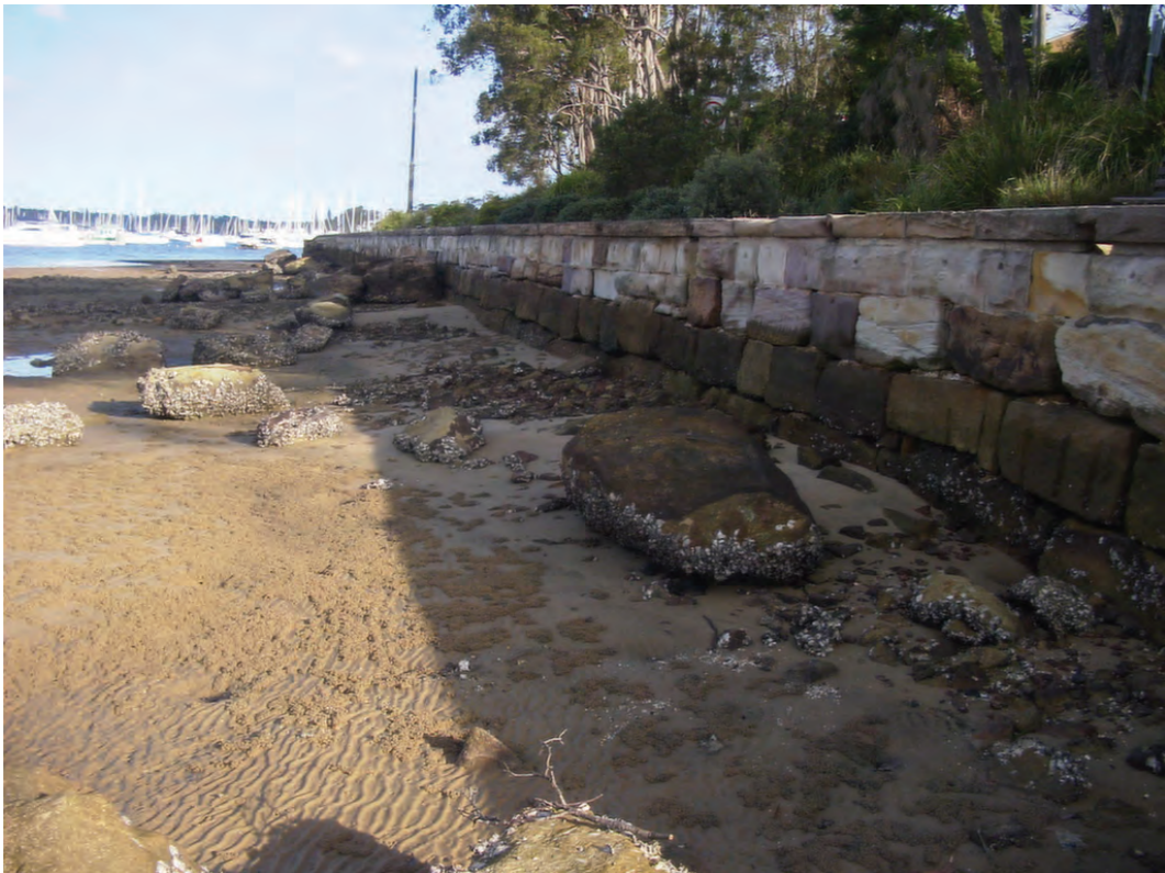
Fig 23 Seawall treatment with large rough faced sandstone blocks and large inter-block crevices, provision of rock rubble at the toe of the wall and retention plus placement of larger rocks off the wall to provide additional hard substratum habitat and shelter.
