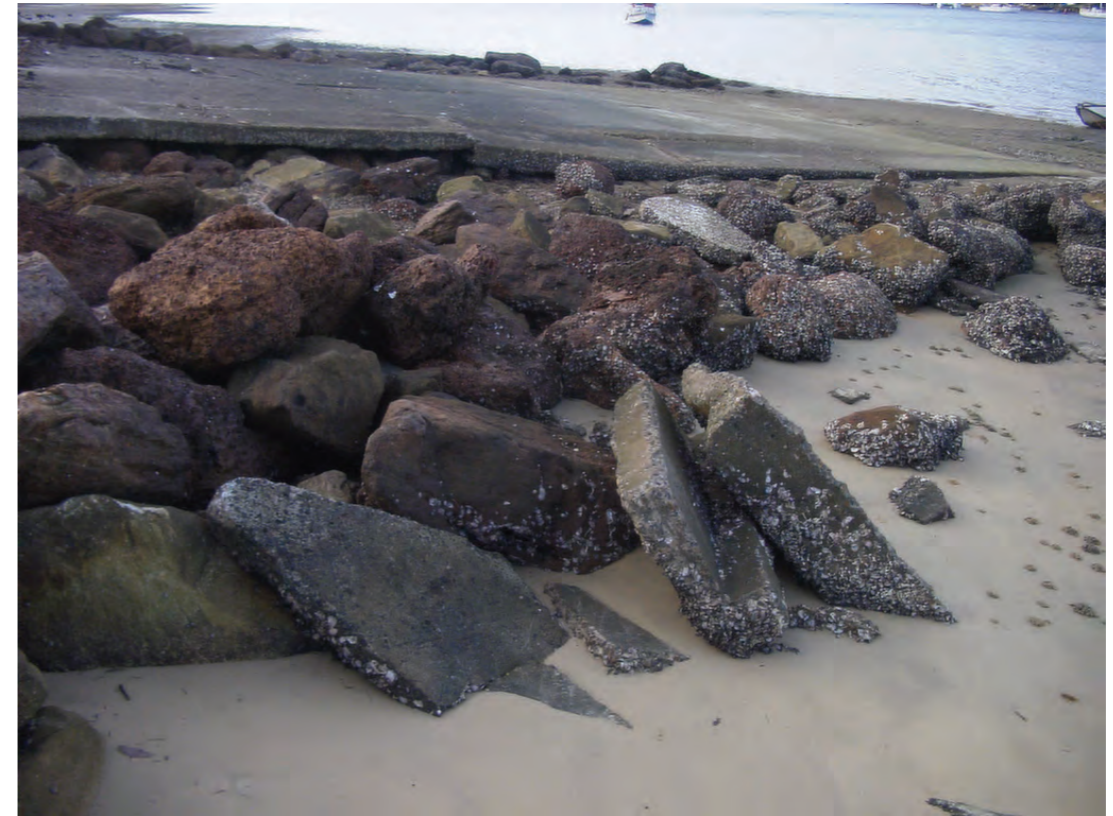
Fig 5 Lower end of Boat Ramp with concrete and rock rubble on sand
