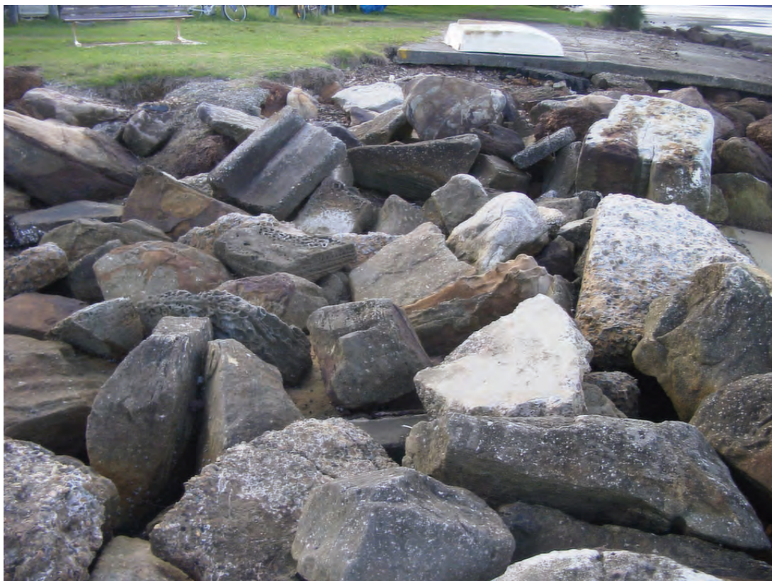
Fig 4 Upper end of Boat Ramp showing mixed rock, tar and concrete fill rubble
