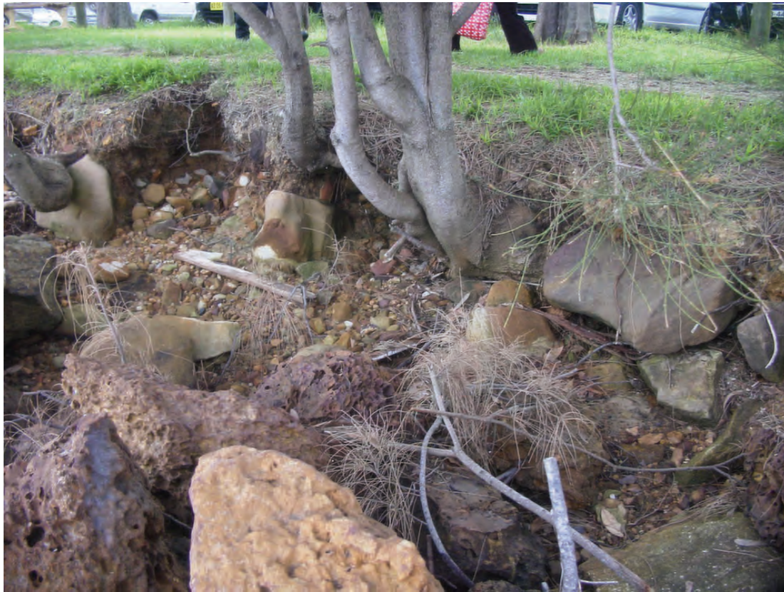
Fig 14 Active bank erosion of an area located between self-seeded She-oaks
