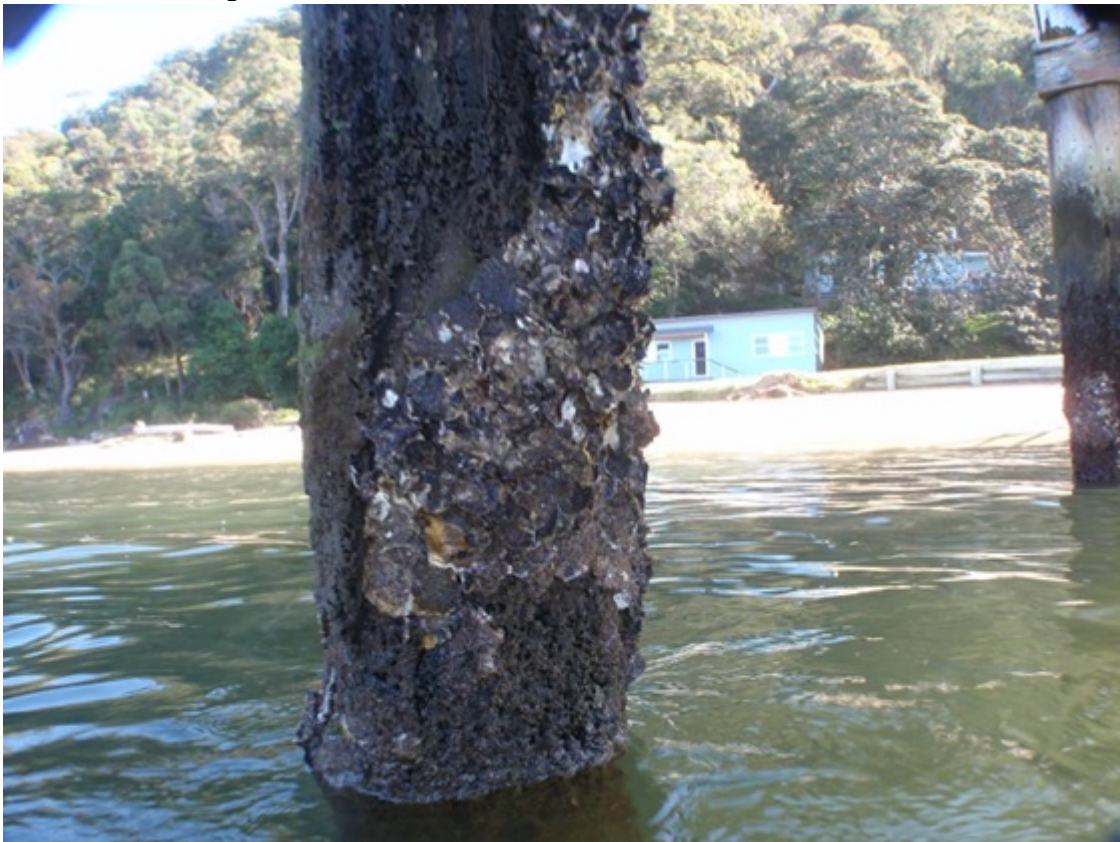
Figure 14 Intertidal oyster band on timber support pile.
