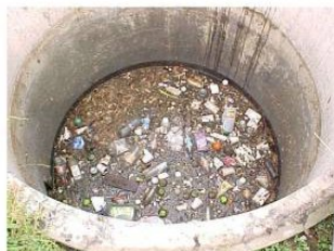
Photo 2. Gross Pollutant Trap at Kitchener Park.
